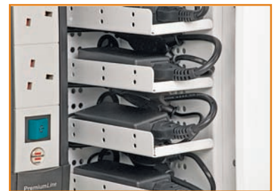
Power pack shelves located in the rear compartment provide excellent cable management
