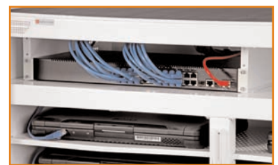
19" rack for mounting a network switch and facilitating data transfer activities
