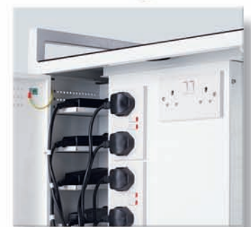
Power pack shelves improve accessibility and cable management
