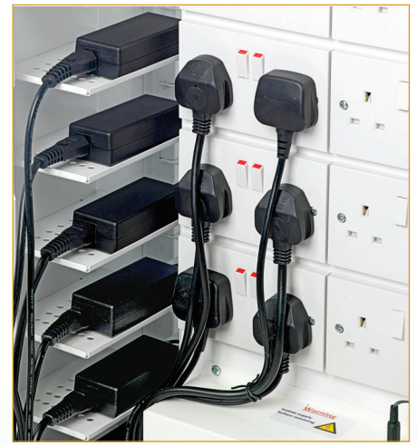
Power pack shelves & Y-leads provide excellent cable management and ease of use
